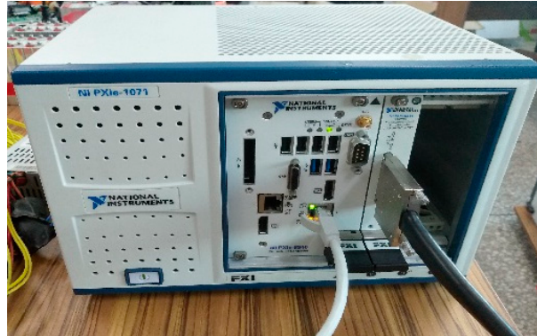
Figure 25. NI data acquisition system.
